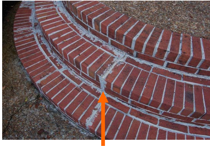
Crack that has been repaired
