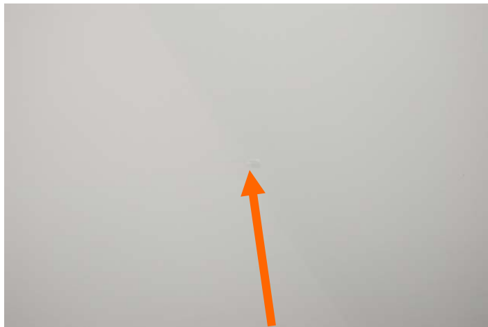
Nail backing out
