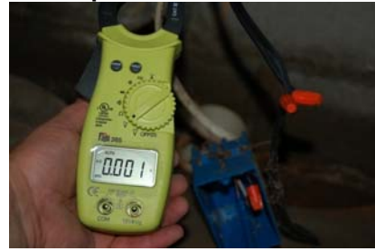
Open box and bare wires in crawl space but did not appear to be connected to electricity
