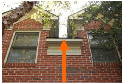
Gutter missing (may be by design)
