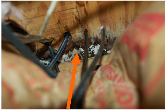
Moisture damage, may be from drilled holes
