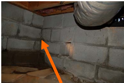
Common mortar joint moisture
