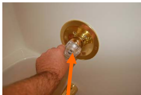
Handle loose and missing the center screw cover
