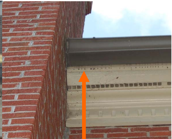
Gutters do not have an end piece or is leaking
