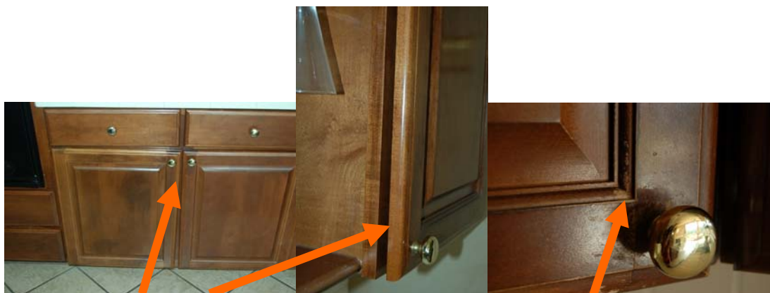
Cabinet doors need adjustment
