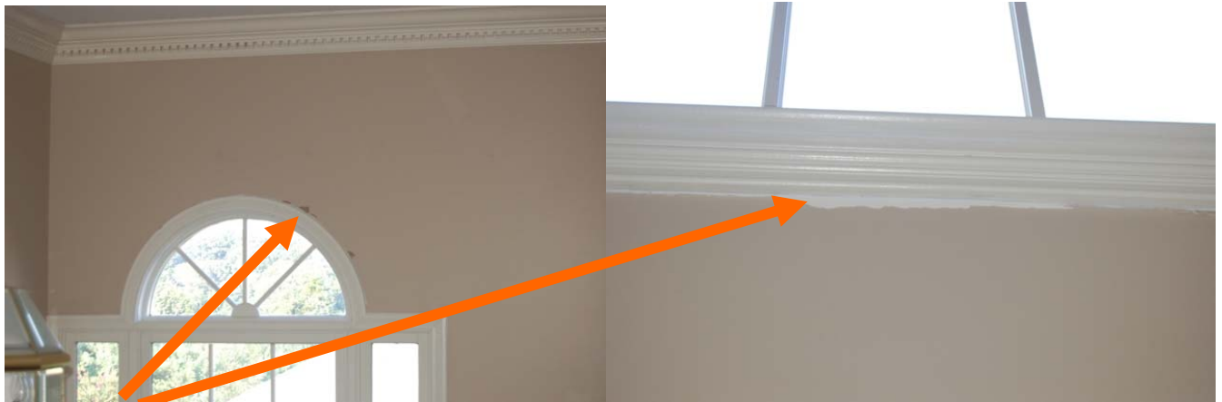
Uneven or missing paint.
