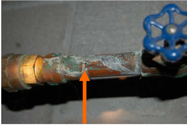
Typical copper corrosion
