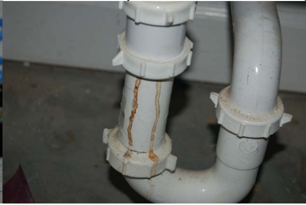
Evidence of old leak in garage sink drain (appears to have been repaired)
