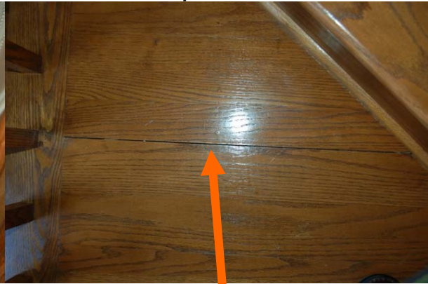
Cracks in stairs
