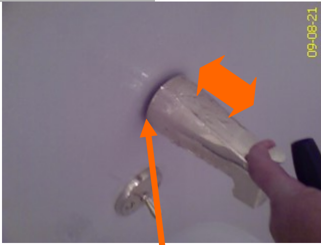
Faucet needs to be secured; movement can cause leaks behind the wall.
