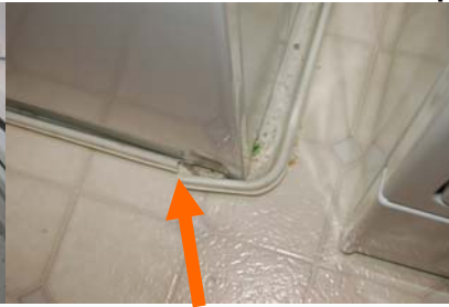
Cracked washer pan
