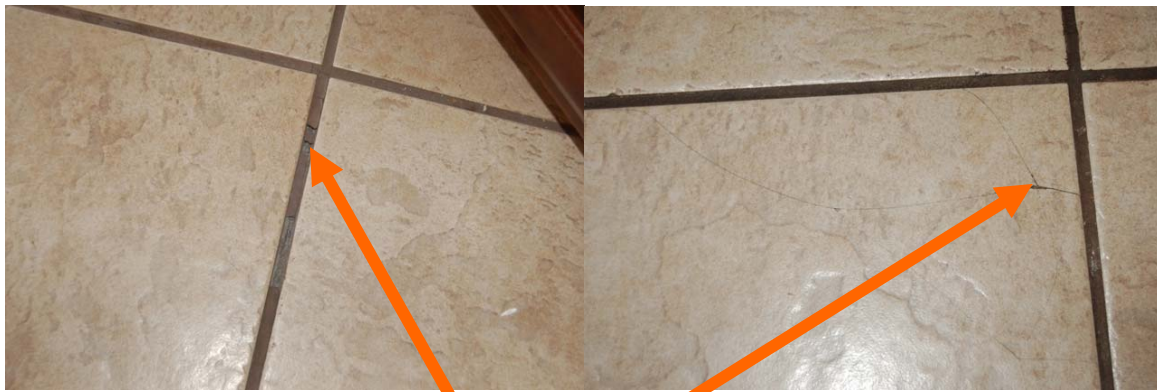
Grout coming out and tile is cracked.
