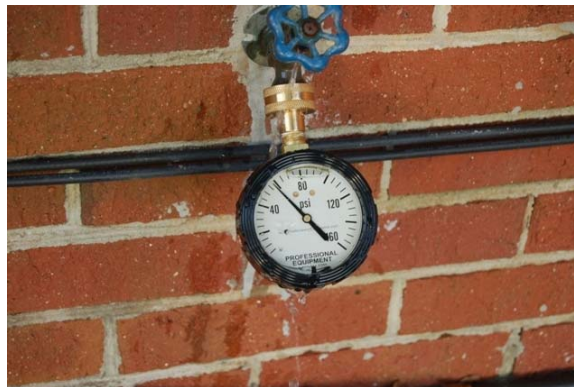
Satisfactory water pressure
