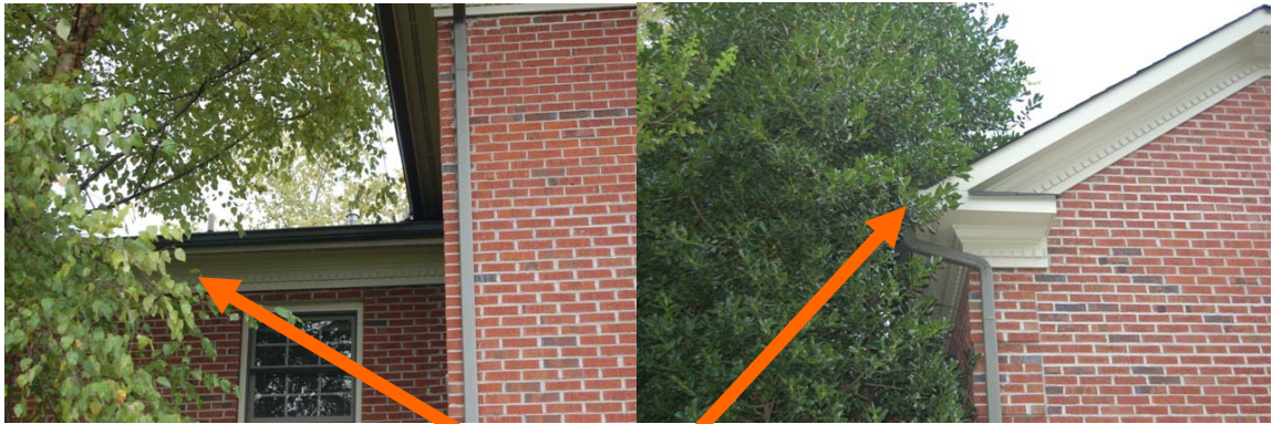
Trees need to be trimmed away from the house.
