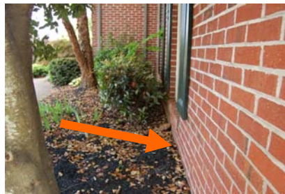
Negative slope under missing section (could lead to water drainage problems)
