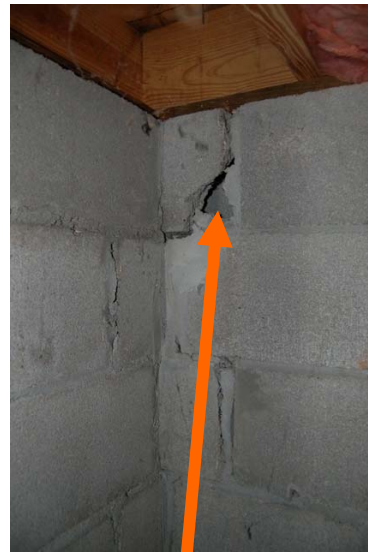
Poor mason workmanship (does not appear to have caused foundation problems)
