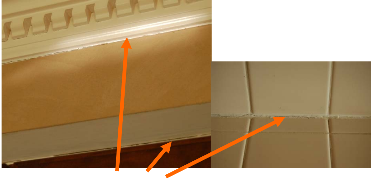
Trim and countertop needs to be recaulked (this is common)
