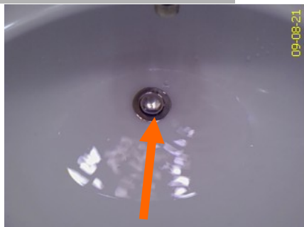
Drains show sign of back-up
