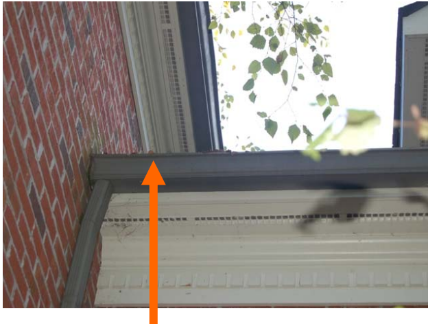
Gutters need to be cleaned
